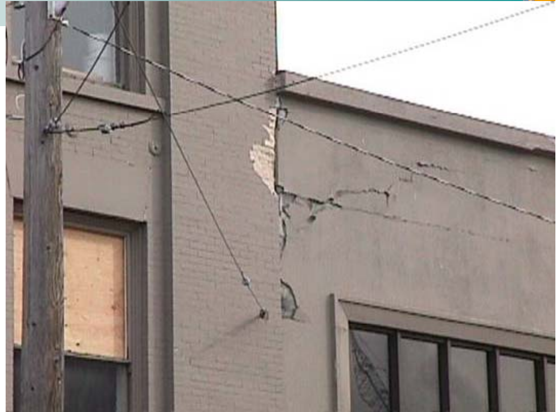
28 February 2001, Mw 6.8 Nisqually, Washington Earthquake
